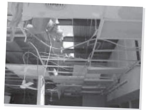
Aurora Pharmacy's roof, ceiling tiles and light fixtures were gone, and drugs and other merchandise were destroyed by the water damage from the storm.
