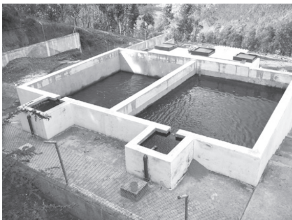
Water flows by gravity from an underground spring into three holding tanks where it is chlorinated.
